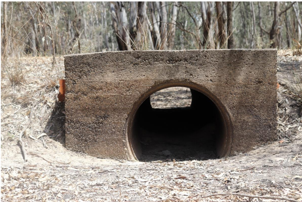
Figure 16: Road culvert acting as a floodrunner constraint.
